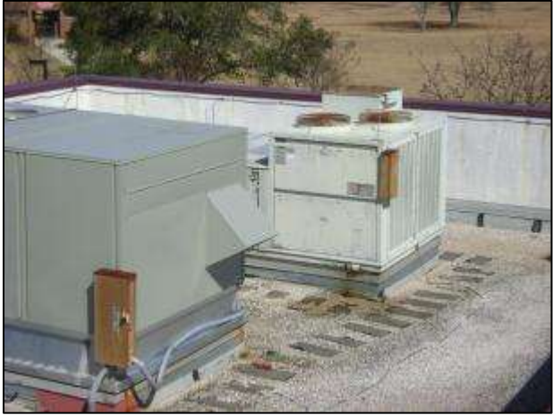
Aerial view of existing 25 Ton RTU to be replaced
