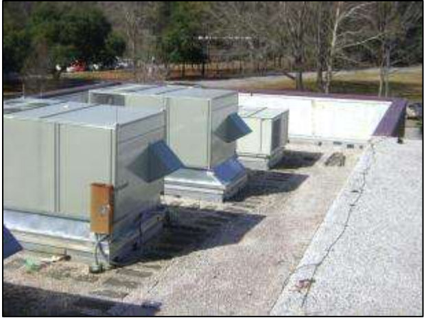
Aerial view of existing 20 Ton RTU to be replaced
