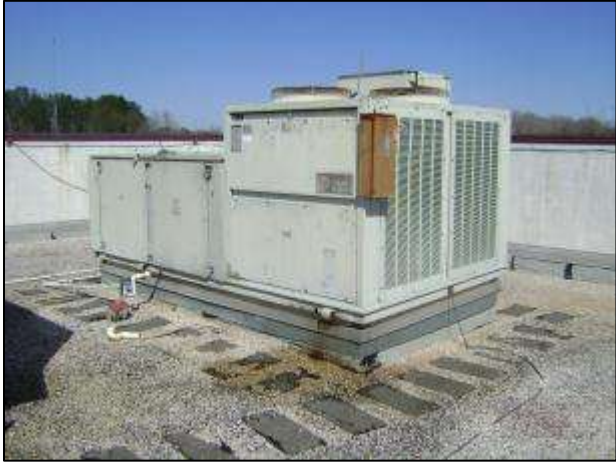
Existing 25 Ton RTU to be replaced
