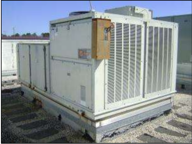
Existing 20 Ton RTU to be replaced
